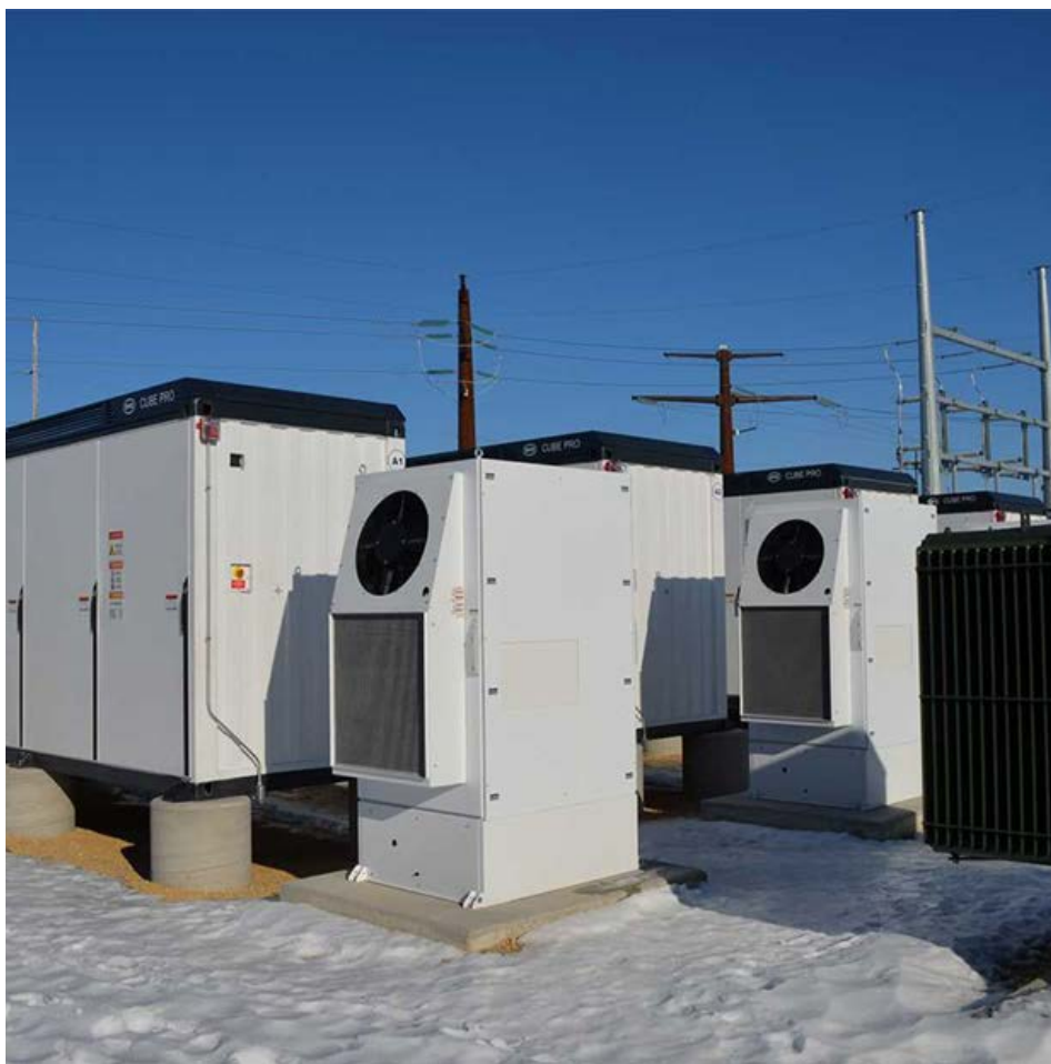
Alliant Energy battery storage in Portage, Wis. | Alliant Energy
